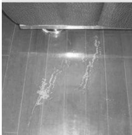
Scratched Wooden Floors
